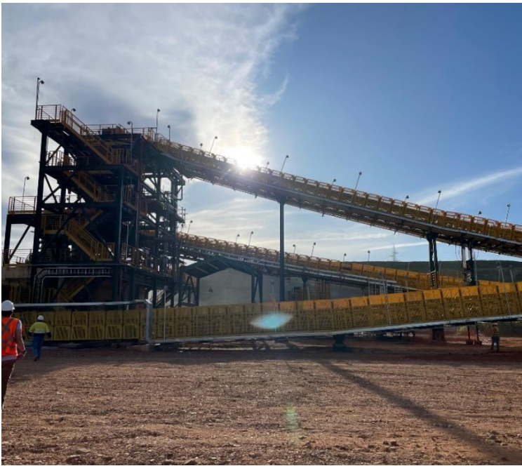
Figure 1: Commissioning of crushing circuit now complete
